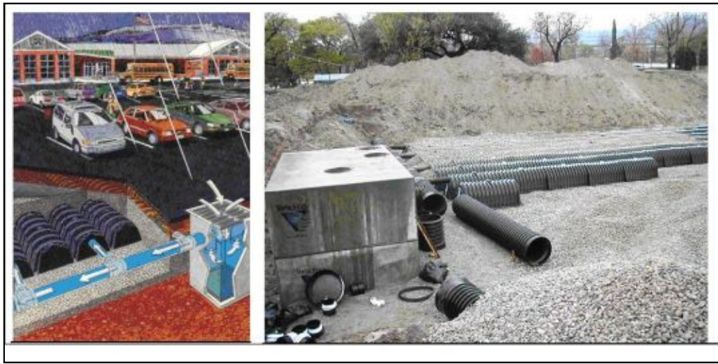
Figure 3-15 Subsurface Infiltration Devices
